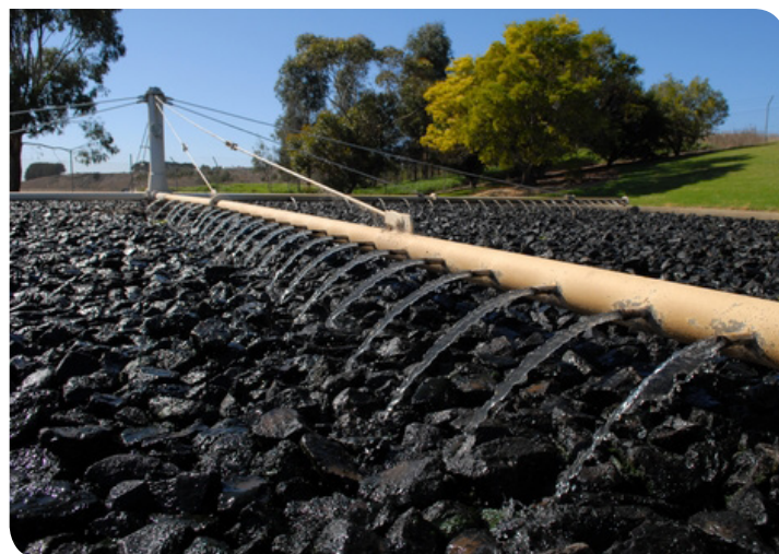
Trickling filters at the Camperdown Water Reclamation Plant
