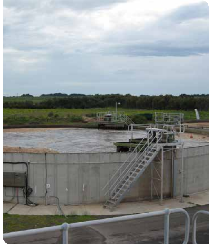
Sewage being treated in the Intermittently Decanted Extended Aeration (IDEA) process at the Port Fairy Reclamation Plant
