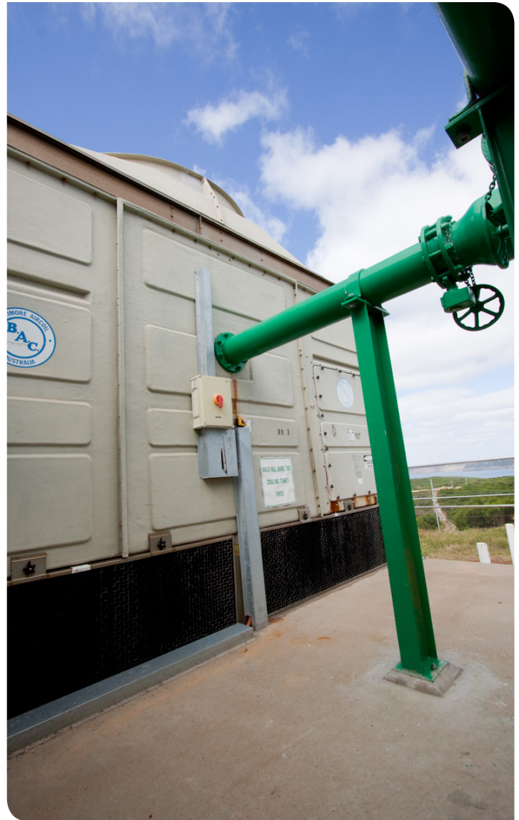
Cooling towers at the Portland Water Treatment Plant
