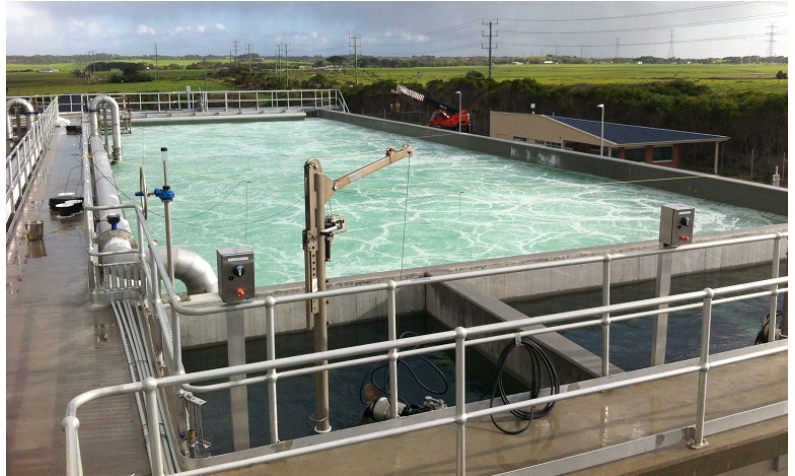
The aeration lagoons at the Portland Reclamation Plant
