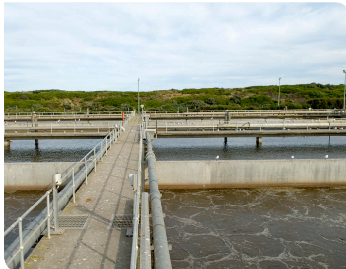
Activated sludge tanks at the Warrnambool Reclamation Plant
