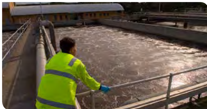
An activated sludge tank at one of Wannon Water's Reclamation Plants
